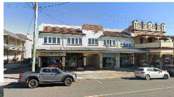
214 DOWLING ST CANTILEVER COMMERCIAL AWNING. EXPOSED STRUCTURE. NO HERITAGE FEEL. STORM WATER RETICULATION ON DISPLAY.
