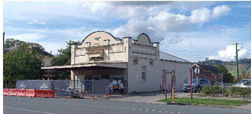
243 DOWLING ST COMMERCIAL CANTILEVER AWNING CURRENTLY UNDER RENOVATION SHOWING ISSUE WITH THIS TYPE OF AWNINGS AND MAINTENANCE
